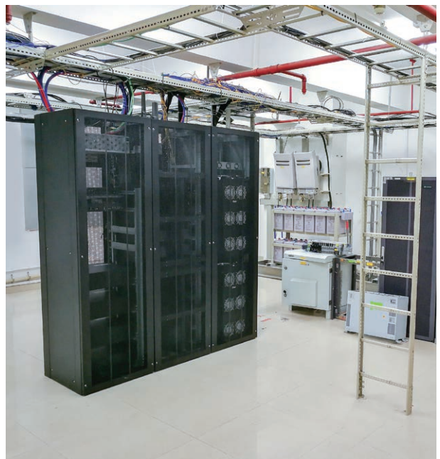
Figure 5 - Simplified Equipment room
