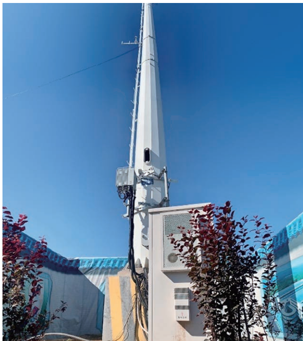
Figure 3 - One Site One Cabinet
