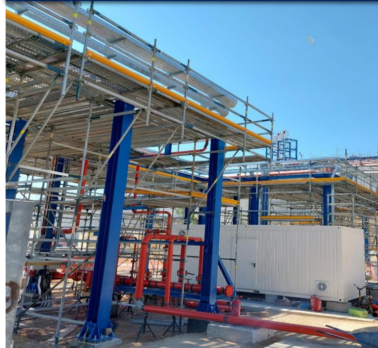
Electrical & Instrument Container (The Control Room)
