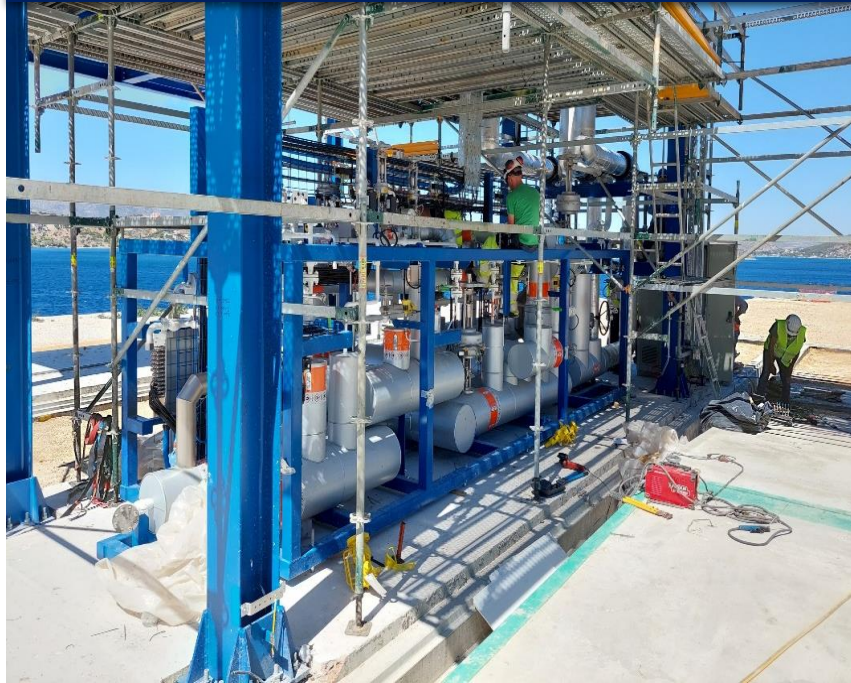
Truck Loading skid (The place of the Loading)
